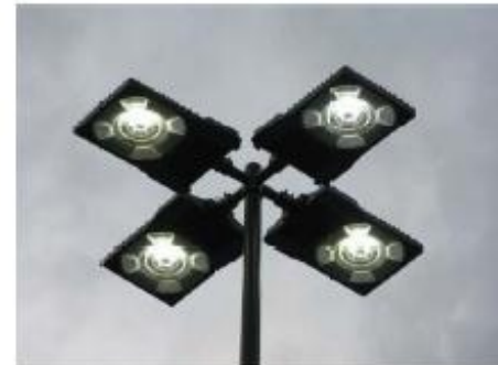
Figure 2.8. GE luminaires on top of poles
